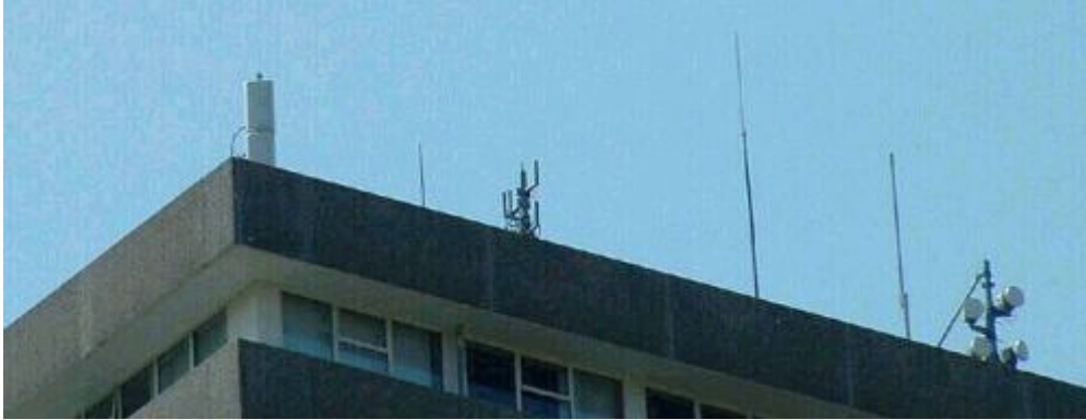
Figure 3.2 DVB-T antenna on the roof of a building in delft source: [28]
